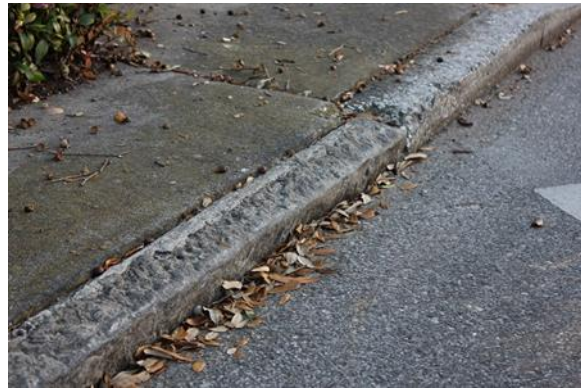
Inconsistent granite curbing 1 st Avenue North
